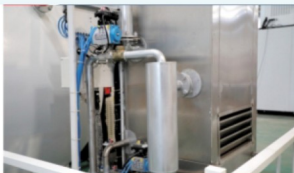
Water Cooling System
